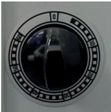
Timer on the contactor box
